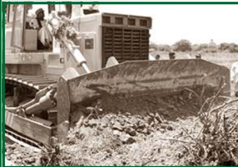
Chief of Presidential Special Task Force on Rehabilitation and Resettlement of the North and parliamentarian Basil Rajapaksa at the controls of an earth moving machine
